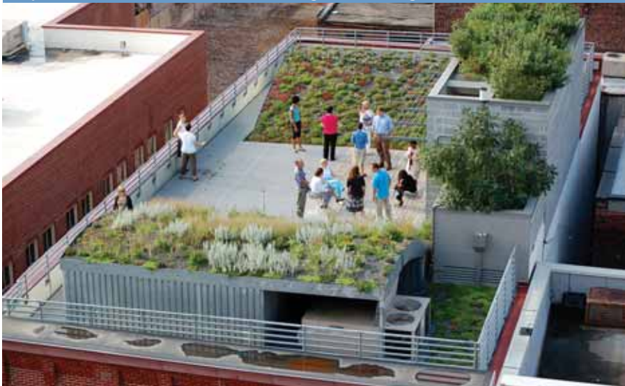
A view of the green roof at the American Society of Landscape Architects headquarters, Washington, DC. The mounds are filled with rigid insulation to reduce weight while enhancing the visibility of plants from the street. The grated walking surface beyond the deck has Sedum growing below it for additional roof plant coverage.
