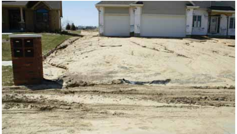
Strict regulations and fines are now in place to help ensure that the lack of erosion and sediment controls on this site is not ignored.
