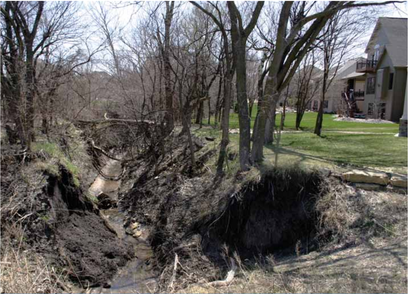
Concentrated stormwater runoff, as a result of impervious surface construction and other changes to the developed land hydrology, has led to significant erosion and pollution problems along virtually every urban and suburban stream and water body.
